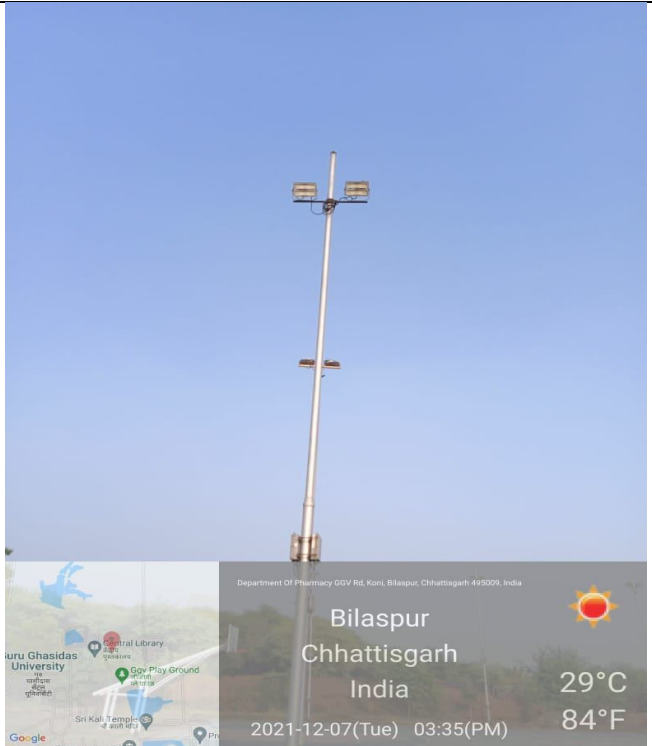
LED flood light in university Sports arena
